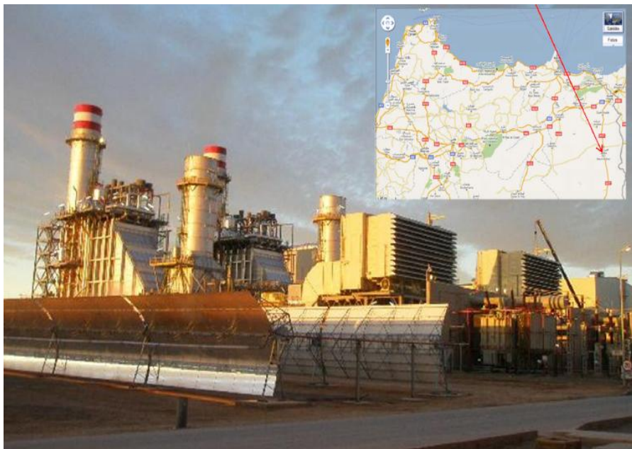
Figure 5 – Centrale hybride CSP – gaz de Ain Beni Mathar, Maroc
